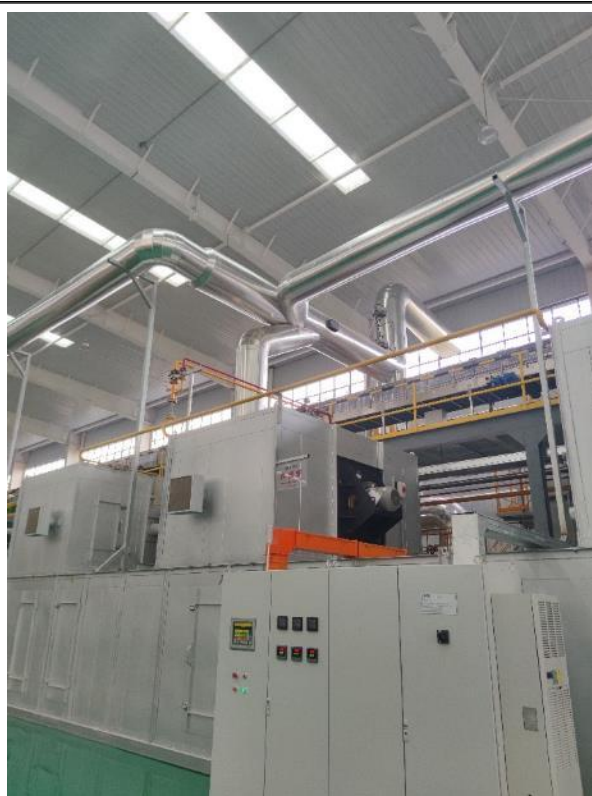
干式过滤+沸石转轮浓缩+ RTO 燃烧
